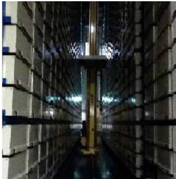
AS/RS rack structure
