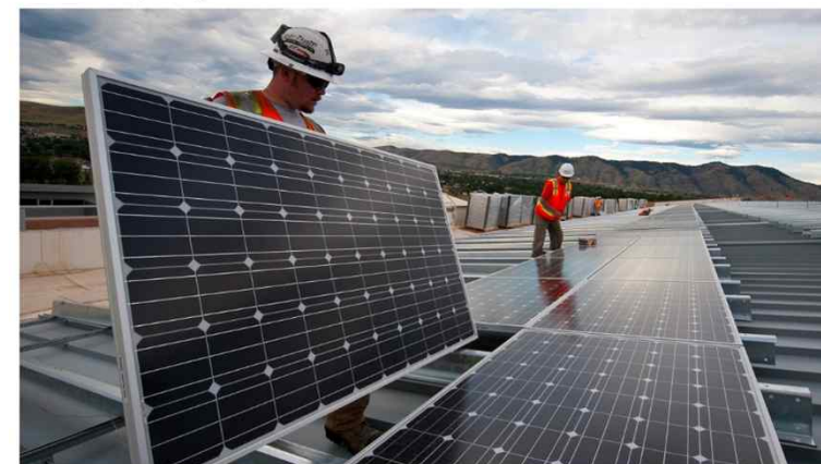
© Shutterstock/Michel Luiz de Freitas | Workers install solar panels in Rio de Janeiro, Brazil.
